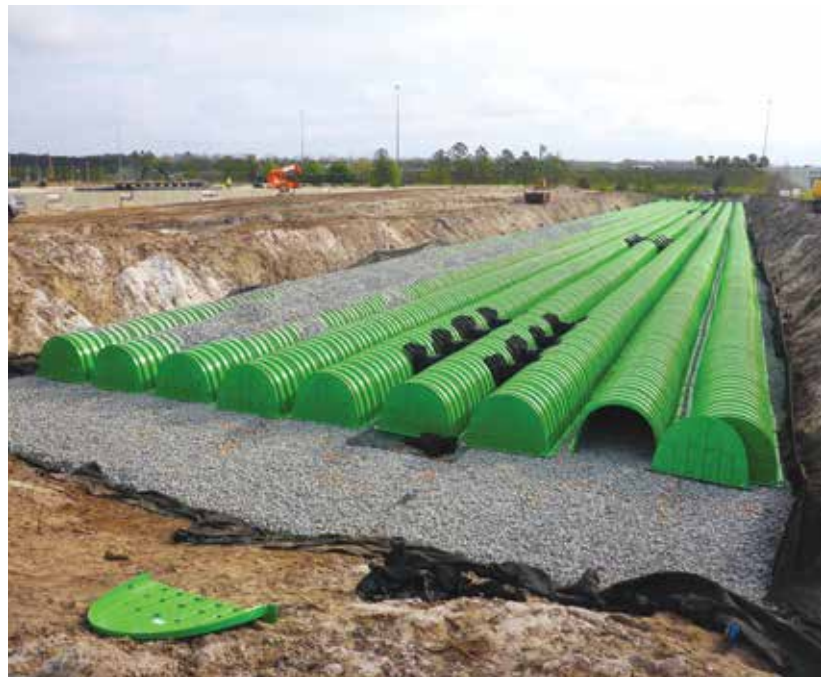
The use of Triton chambers allowed the development team to do less excavating and use less crushed stone — saving money in all phases of the project!
