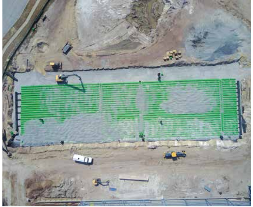
Triton M-6 Chambers were used in Basin 2. The basin relied on a combination of Main Header Row technology and direct input into the distribution rows to manage flows from parking lot drainage and roofline runoff.
